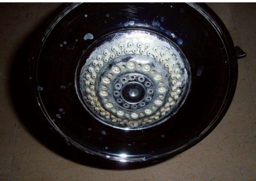
Figure 4 Scale buildup on hotel showerhead
