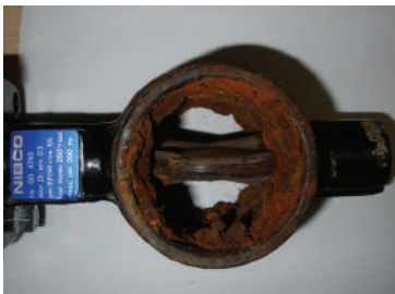
badly scaled valve Feb 2009
