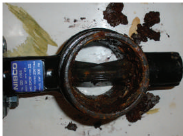
11 weeks after Aqua-Rex was installed
